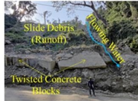
Left flank of the slide at road level
